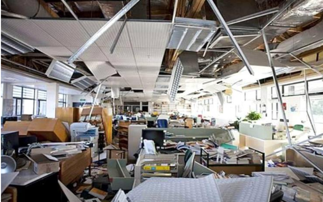
Figure 3: Ceiling damage from the New Zealand 2010 earthquake [5].
