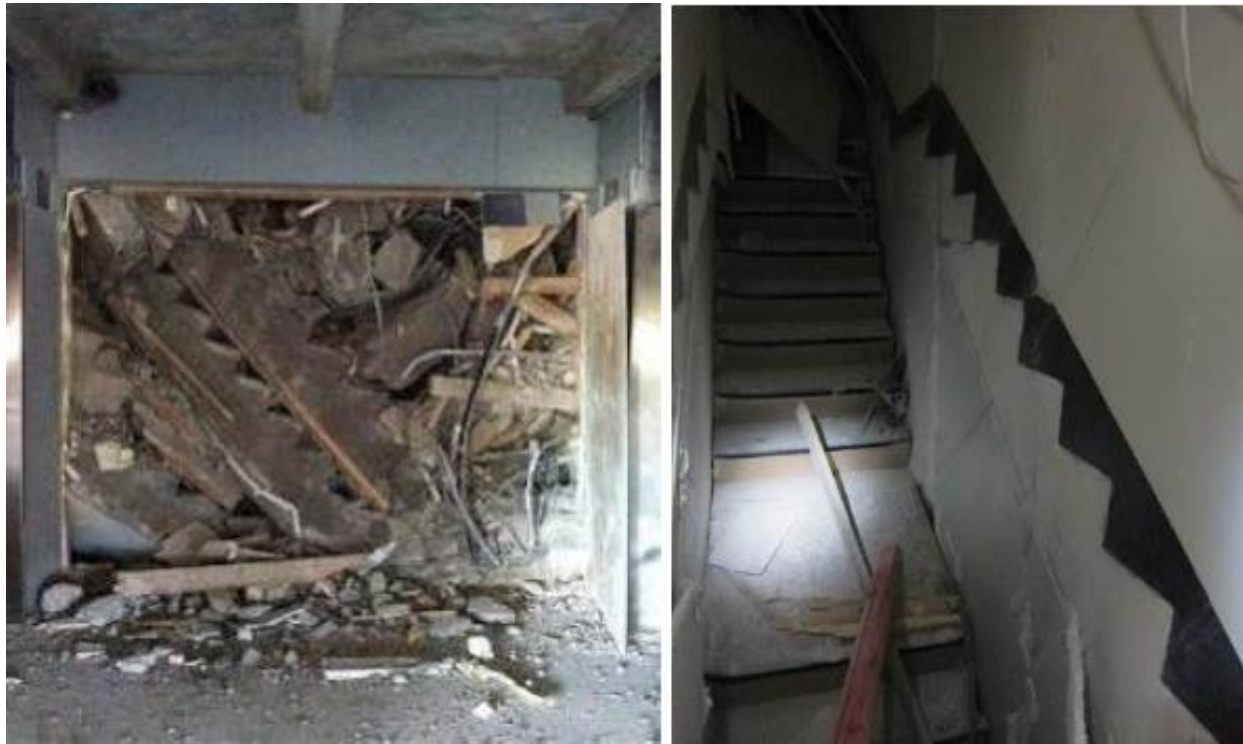
Figure 4: Staircase damage from the New Zealand 2011 earthquake [6].
