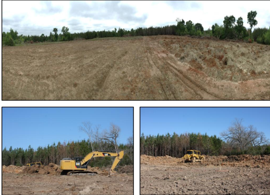
Figure 4. Photos of installation of treatment plots from January 26 to February 1, 2016. Top = from left to right - control, scraper and FRA plots; bottom left = digging to a depth of 1.3 m to simulate mining; bottom right = soil replaced back in 15 cm layers to simulate scraper-pan reclamation.
