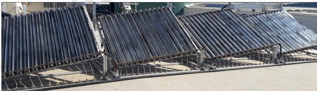
Fig. 3. Image of the thermal solar system.
