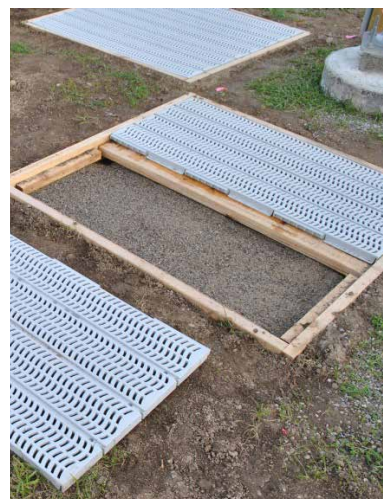
Figure I-1.2.3 A perforated and textured grey plastic target construction. Landscape fabric (thick textile) is installed beneath the target to minimise vegetation growth (Source: ECCC).
