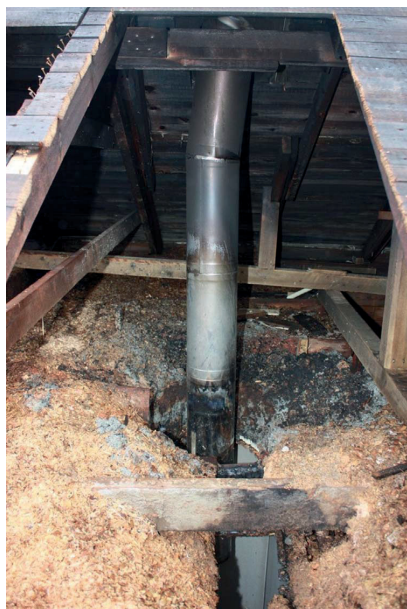
Fig. 1. Chimney roof penetration after fire.
