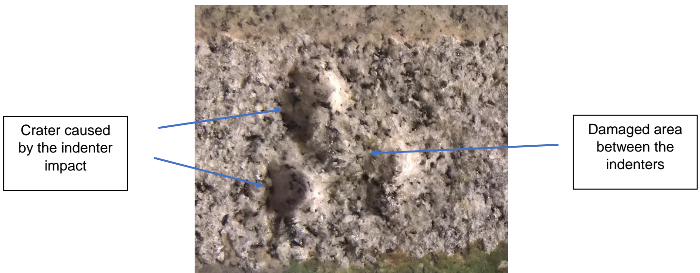
Figure 37 Damaged area on the surface of a 6 second heat shocked block sample of Kuru Grey.
