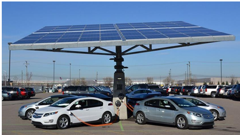
Figure 2.2 Electric vehicles charging station [16].
