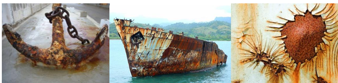
Figure 14. Various structures suffering from corrosion: anchor, vessel and painted surface. (Vincentz Network GmbH & Co. KG, 2011)
