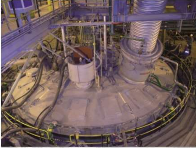
Figure 3. Modern DC-furnace by SMS-Siemag [18]
