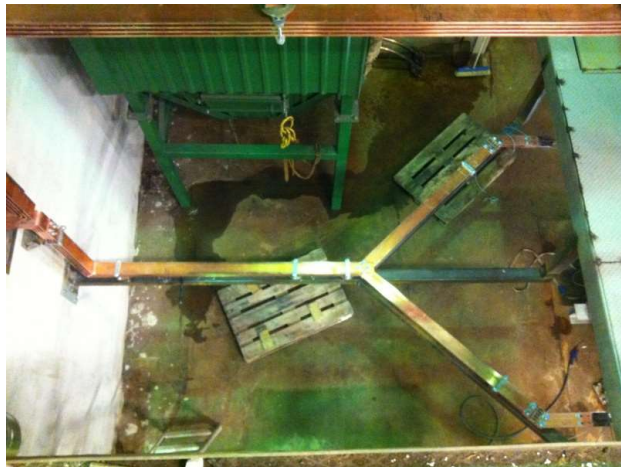
Figure 20. Bus bars coming from rectifier room to furnace
