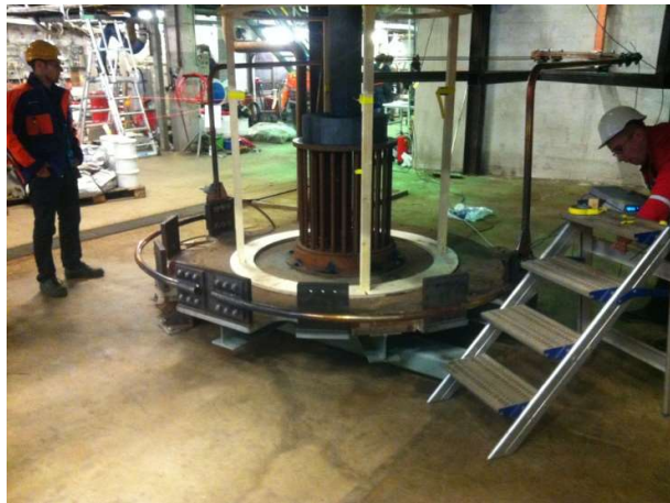
Figure 19. Connection of bus bars to anode and the anode pin
