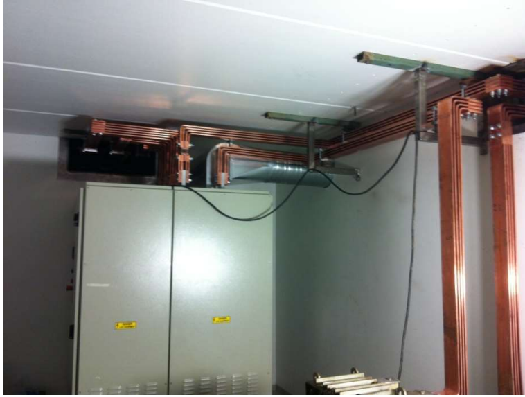
Figure 17. Rectifier connected to bus bars
