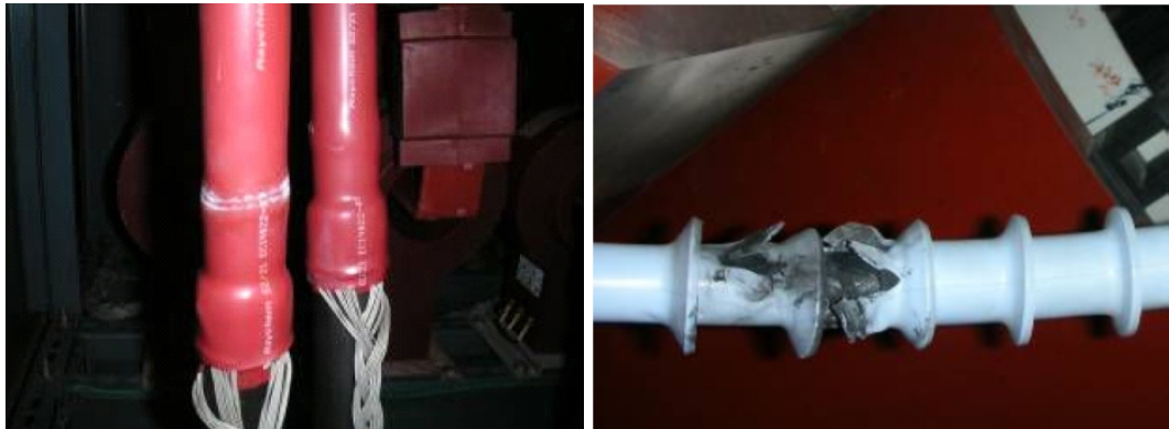
Figure 3.8. Surface discharge ring on top of termination probably due humidity and dirt (left) and high impedance fault in termination (right) [25]
