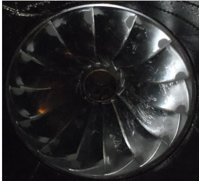
Figure 1.1. Cavitation erosion damage in the Imatra power plant G2 unit runner blades.
