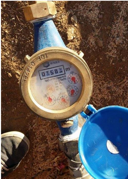
Fig. 5-5. Working water meter (Salmivirta 2015).
