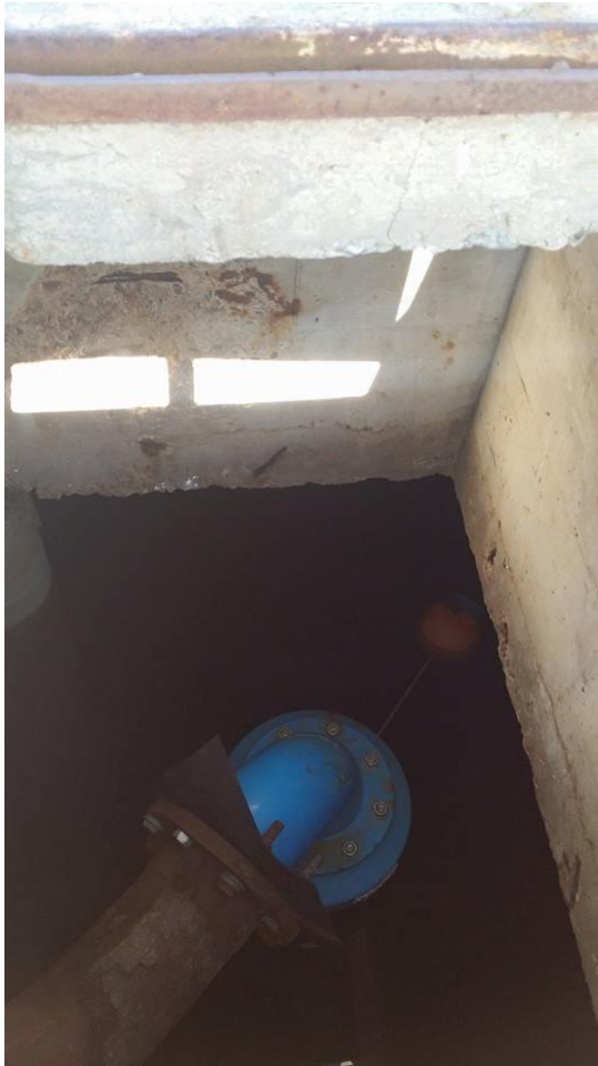
Fig. 5-7. Old float valve in Oypass Hill reservoir (Salmivirta 2015).
