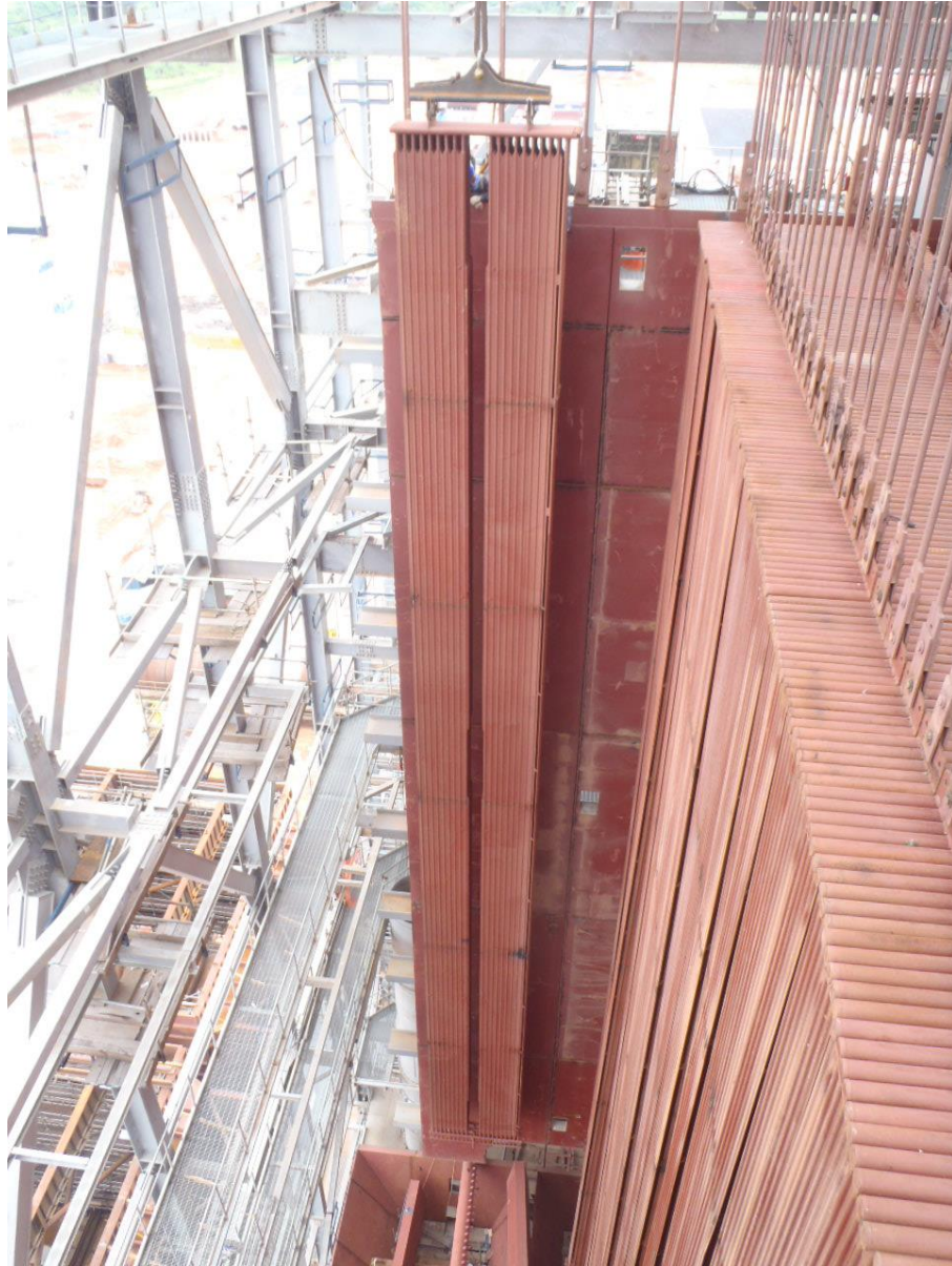
Figure 2. Economizer installation, Valmet Technologies Oy
