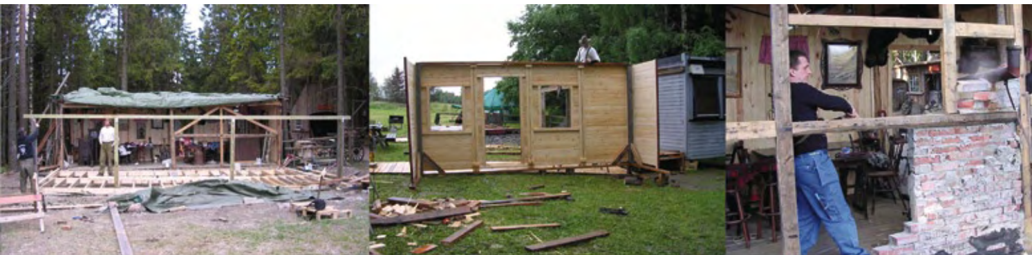
The hardest-working volunteers put hundreds of hours each into building the town. (Construction, Asbjørn Rydland)
