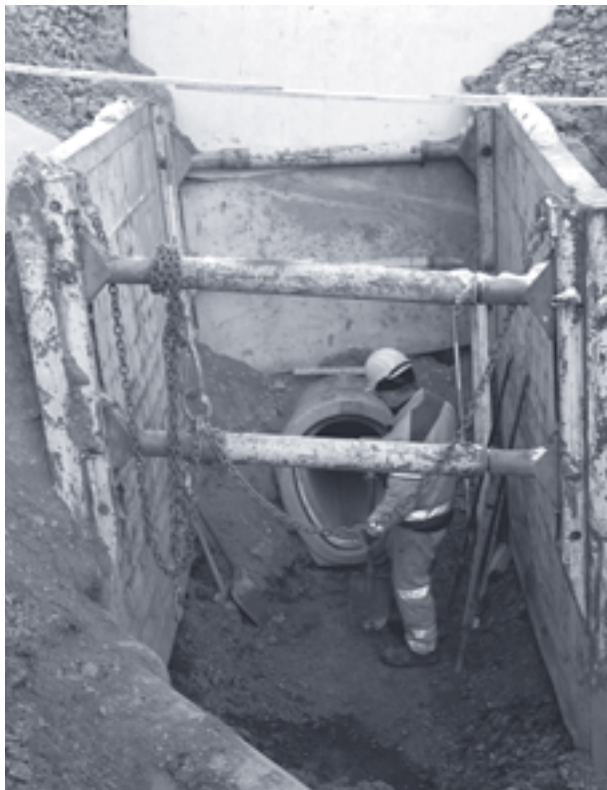
Fig. 7.3 Installation of pre-fabricated concrete gravity sewer of oval shape in the suburb of Hervanta, Tampere in December 2006 (Photo: T. Katko).
