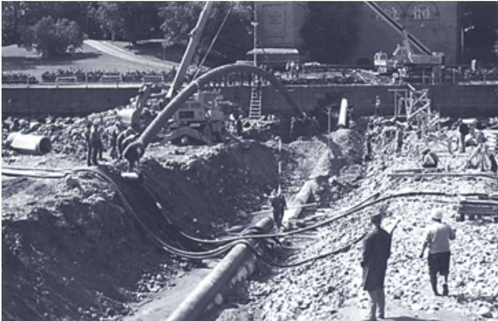
Fig. 5.1 Construction of water pipe and sewer mains under the Tammerkoski rapids in summer 1973 (Photo: Tampere Water).
