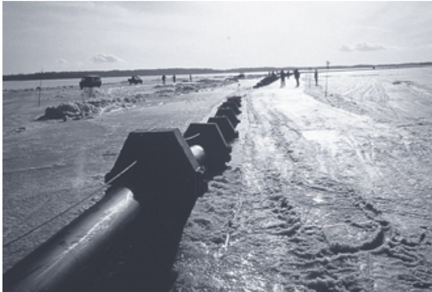
Fig.9.3. Construction of a submerged pressure sewer of PEH on the ice of Lake Pyhäjärvi for bringing wastewaters from Pirkkala municipality to Rahola wastewater treatment plant in Tampere in late winter of 1995 (Photo: Tampere Water).
