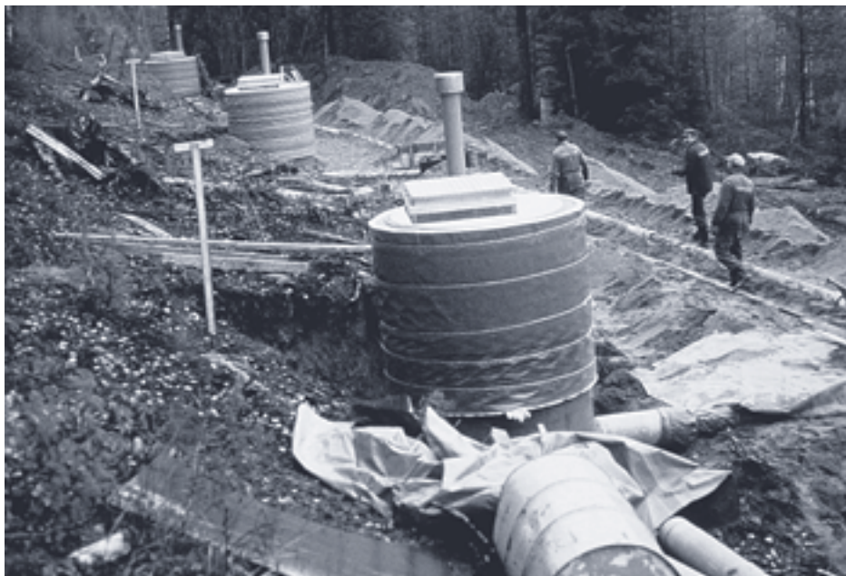
Fig. 4.9 Series of tube wells under construction in Julkujärvi, west of Tampere, in the late 1970s (Photo: J. Koskinen).
