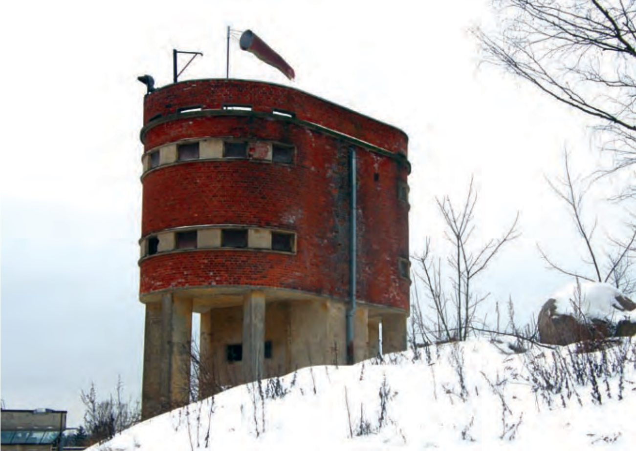
Picture 4. This water tower was used by steam locomotives in Riihimäki. It is not in use anymore. (Juuti 2009)
