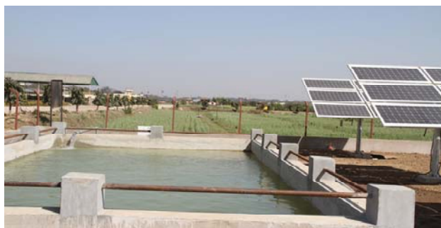
Fig. 16.5. Solar water pumping system installed at Patna
