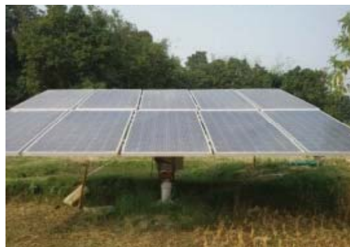
Fig 16.9. Solar groundwater pumping systems at village Bhagwatipur in Madhubani district of Bihar.
