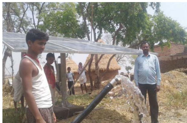
Fig. 16.3. Solar pump at Bharatpura village, Patna
