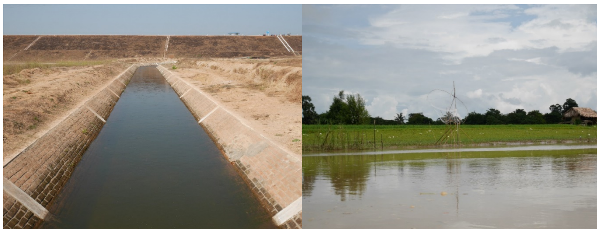
Figure 3.4 Embankments made to the Mazin Chaung in upper parts (upper) and the Eastern bank of the Bago River Between the Bago City and Tawa Village (lower).
