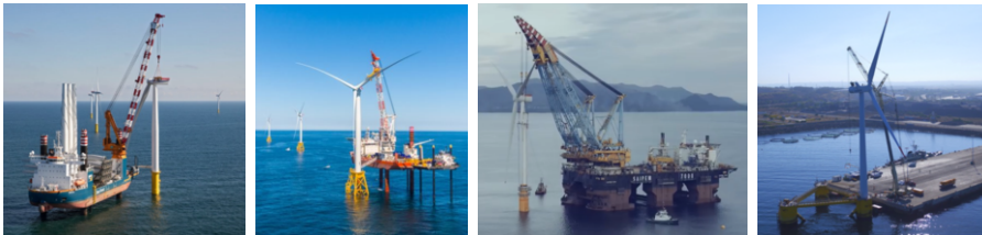
Figure 2.18: Examples of offshore wind farms during installation (from left: Gemini Wind Farm in the Netherland, installed by Van Oord (Irving, 2017); Block Island Wind Farm in the US, installed by Fred. Olsen Windcarrier (Finucane & Hall, 2016); Statoil Hywind Wind Farm in Scotland, during assembly in Norway by SAIPEM 7000 (Statoil, 2017b); WindFloat prototype at Sines quay side in Portugal, under decommissioning (Roddier et al., 2017))
