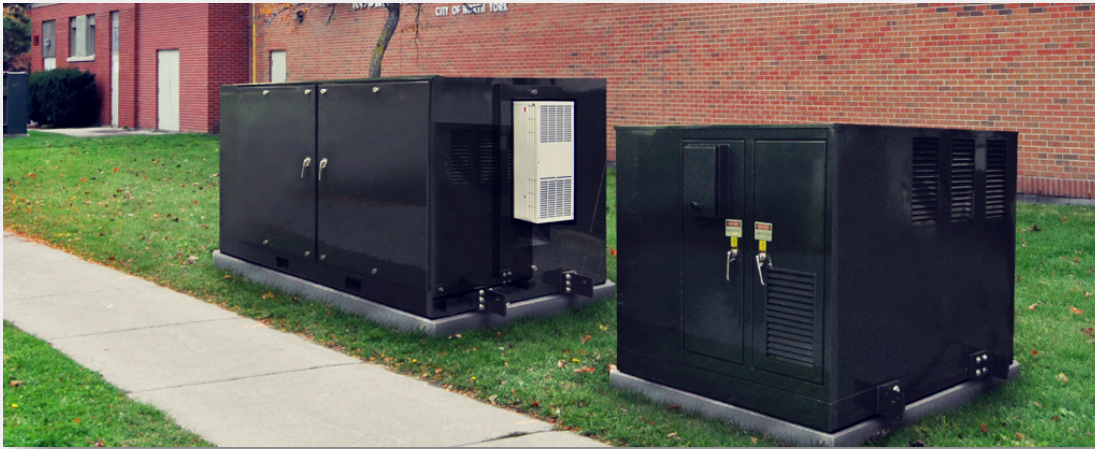
Figure 3.3 This unit will provide 250 kWh/500kW of storage and is very compact; it only requires a small pad mount, a bit larger than a normal Toronto Hydro transformer. (Source: http://www.ecamion.com/ )
