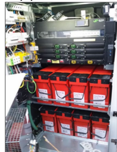
Figure 4.10 Battery system (battery, inverters and local EMS/BMS display) [5]
