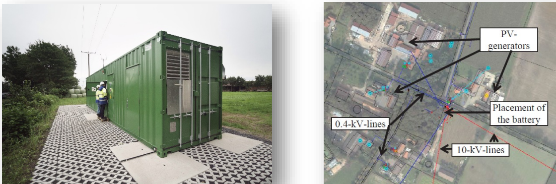
Figure 3.4 The utility scale 250kW/1MWh battery system (left) and the location in Wetringen, Germany with grid assets, farms, and PV-generators (right). (Source: [9])
