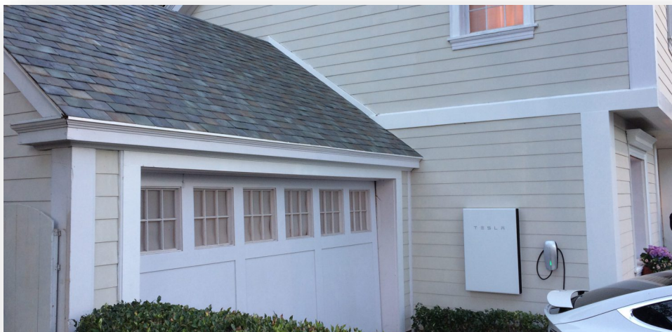
Figure 3.2 Installed Powerwall 2 battery storage system on a residential household (Source: www.electrek.co )
