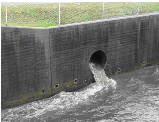
Figure 5 Discharge of untreated stormwater from a stormwater sewer
