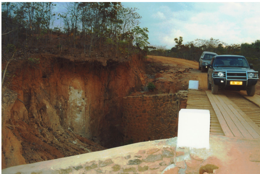
Figure 7. Erosion caused by the construction of a low-cost feeder road in the hills of northern Malawi (photo: K. Esser).
