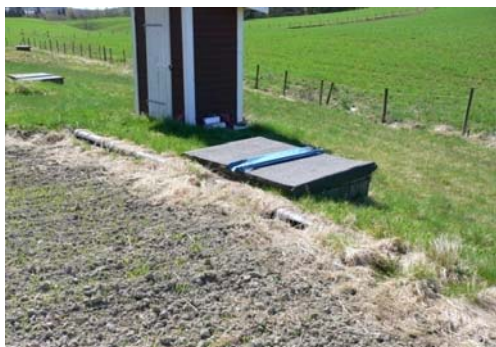
Figure 11. Perforated pipe that collects surface water
