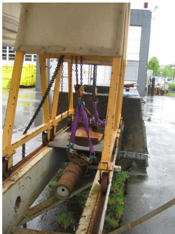
Figure 6-3 Trolley and chain hoists
