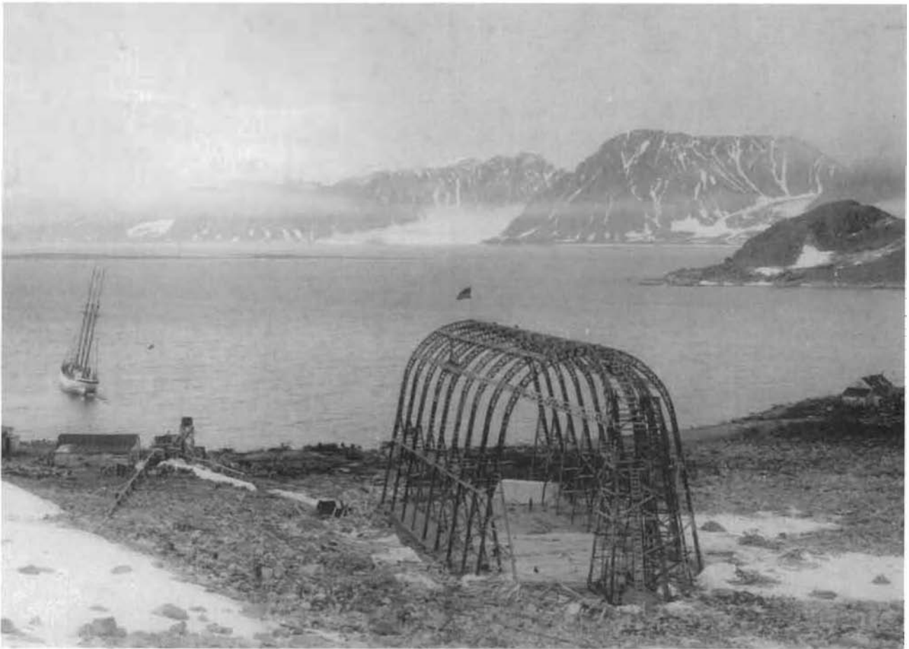
Fig. 23. The airship hangar at Camp Wellman being rebuilt in 1909. Photograph from Wellman's book The Aerial Age .
