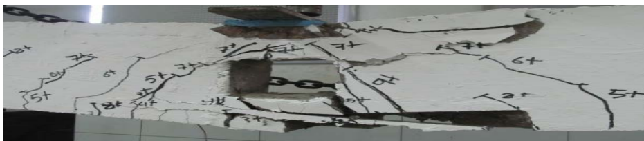
Figure 16: Crack pattern for beam F-L-N
