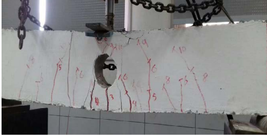
Figure 9: Crack pattern for beam F-C
