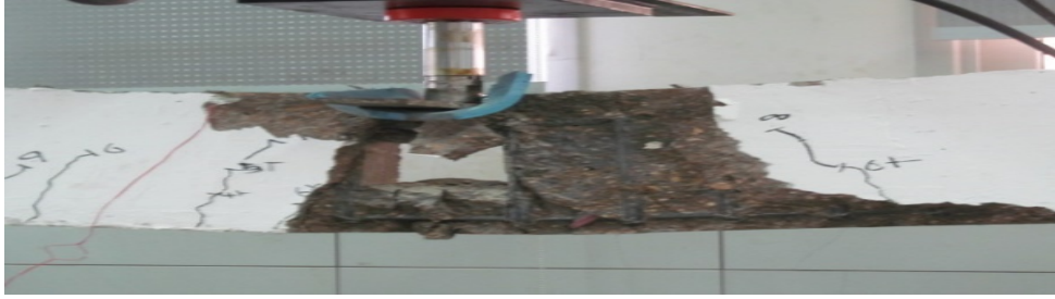
Figure 6: Crack pattern for beam F-S
