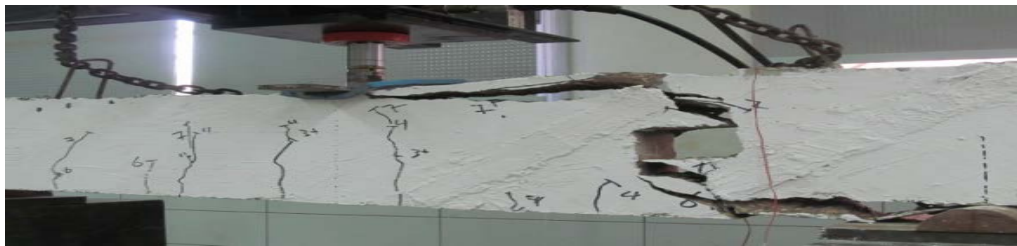
Figure 21: Beam S-L-E Crack pattern
