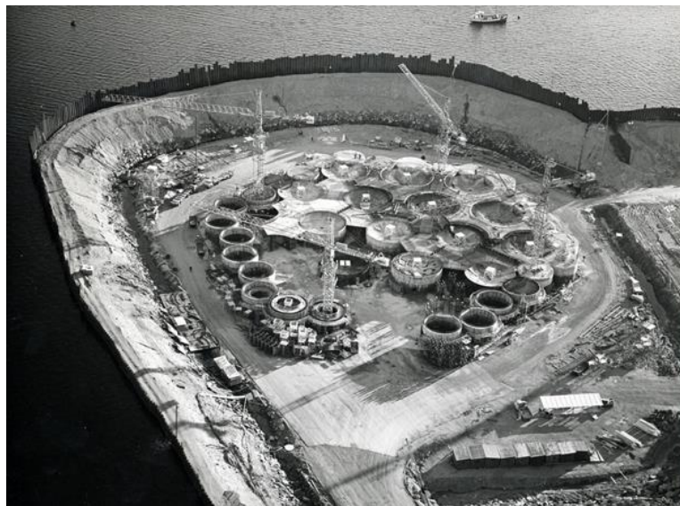
Figure 3-2 Temporary graving dock for the manufacturing of the "Condeep" O&G platform's concrete floater
