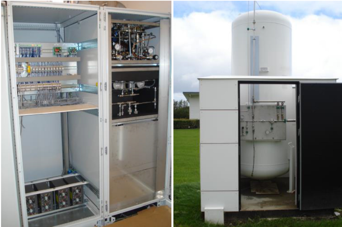
Fig. 27: Left: The electrolyser system used for H 2 -College. Right: The hydrogen storage tank from H 2 -College,
