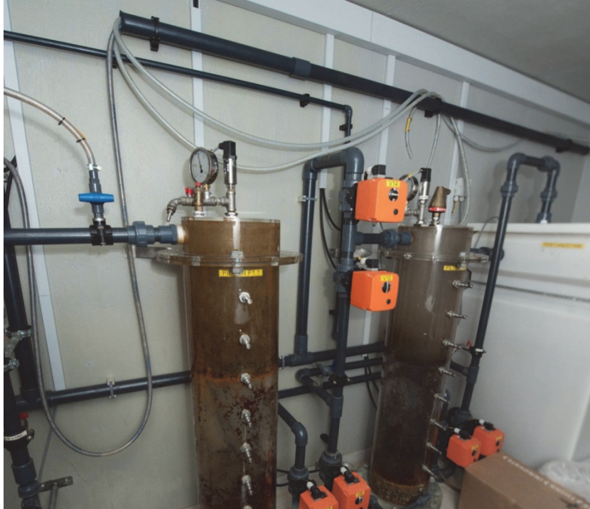
Figure 8. Picture of the two pilot columns used in the study at Islevbro water works (photo courtesy of Philip Binning)
