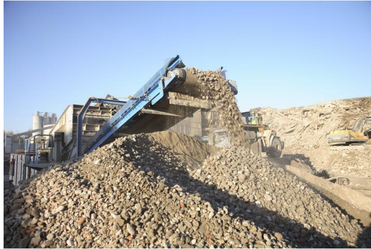
Figure 5. Concrete waste from a selective demolition of constructions has favourable properties for use in road constructions and can replace natural materials. C&D wastes are generated at three types of sites - renovation, demolition and new construction sites. The waste streams of construction sites are mostly clean material surpluses which are not mixed and contaminated. Demolition and renovation waste, on the other hand, is often mixed and contaminated and thus also more difficult to recover. All of these sites produce different types of waste with their own features and environmental properties to be considered.
