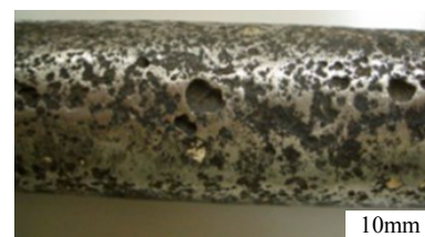
Fig. 2. Appearance of superheater tube Alloy 625 applied for 37,000 h in the Tsukui WTP plant boiler.
