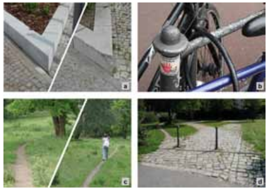
Figure 5: Damage due to design and detailing. a) Damage to acute edging: year 1/year8. b) Damage to bike stand: year 06. c) Visible signs of use: desire paths: year 7. d) Visible signs of use: year 9
