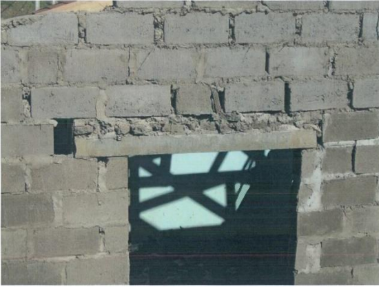
Figure 3: Poor installation of lintel
