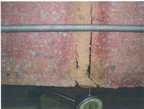
Figure 6: Cracking of unreinforced block beam
