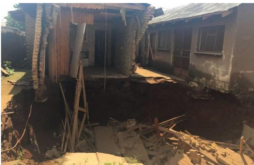
Figure 1: Sinkhole formation on dolomites
