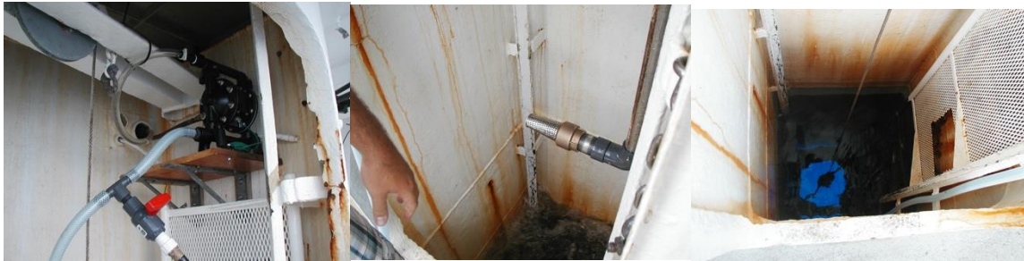
Figure 1. Moon pool aka Straza Tower (center and left), custom intake (center), and the compressed air driven diaphragm pump and hose installed for the flow-through system on the Atlantic Explorer by Norm Nelson.
