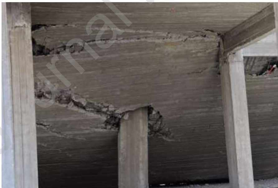
(b) Collapse of residential building in Elshourok city, Cairo (Elshorouk City Website, 2019)
