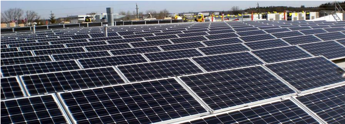
Figure 1-6. A typical solar PV system provided by Enviro-Energy Technologies located in Cambridge, Ontario, with 98,000 kWh electricity generation (Reprinted with permission from Ref. [34]).
