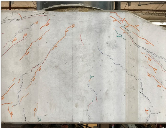
c) Crack pattern at column stub at the 300 kip load case (west face)
