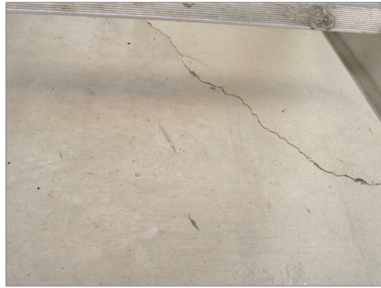
(d) close-up of dominant shear crack (northeast face of BC1)
