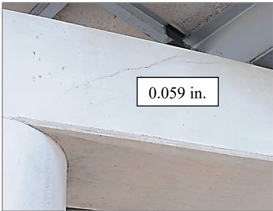
(c) In-field largest width primary crack on SE face of BC2
