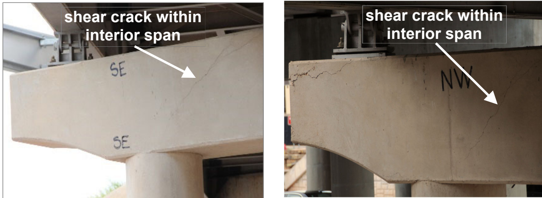
Figure 2.4. Interior span shear cracks
