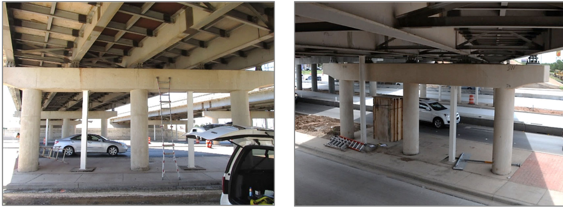
(a) BC1 (west face) (b) BC2 (west face) Figure 2.2. Bent caps while in service
