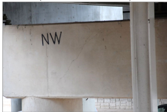
(f) dominant shear crack (northwest face of BC2)
