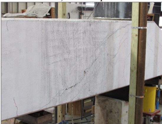
c) Major shear crack on the interior span after test completion (west face)
