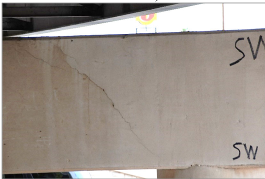
(e) dominant shear crack (southwest face of BC2)
