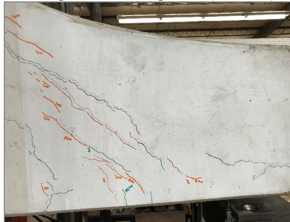
d) Crack pattern at overhang at the 300 kip load case (west face)
