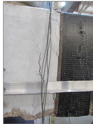
d) Shear and flexural cracks at the face of the column after test completion (east face)
