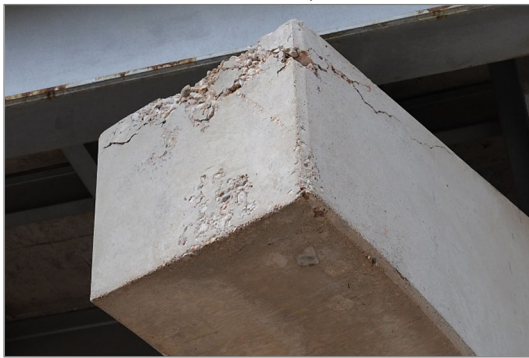
(g) end region cracking, chipping, and spalling (north end of BC2)
