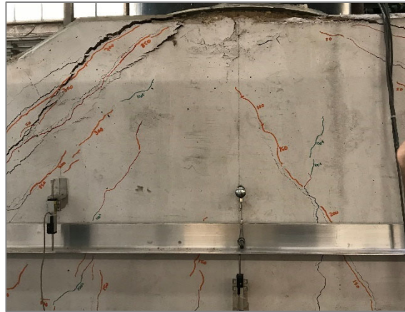
b) Shear cracks and observed concrete crushing after test completion (east face)
