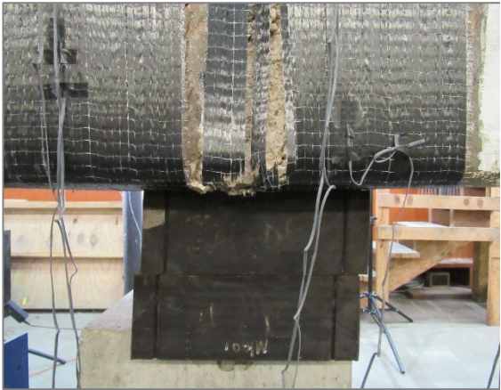
c) Temporary support in contact with bent cap bottom surface (west face)
