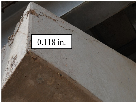
(e) In-field largest width crack on NW face of BC2
