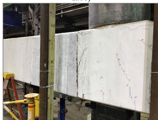
f) Major flexural crack at the face of the column after test completion (west face)
