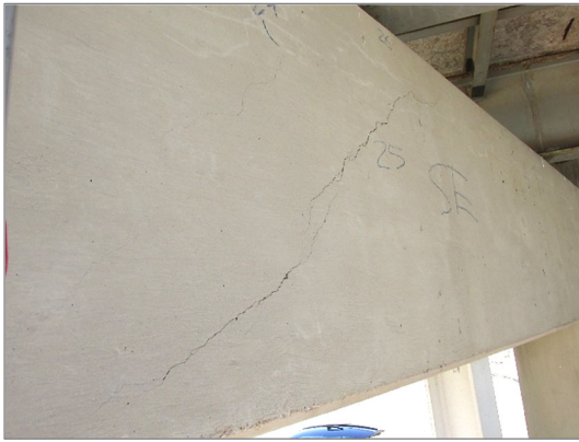
(c) dominant shear crack (southeast face of BC1)
