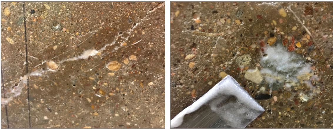
(a) thickened epoxy on crack
