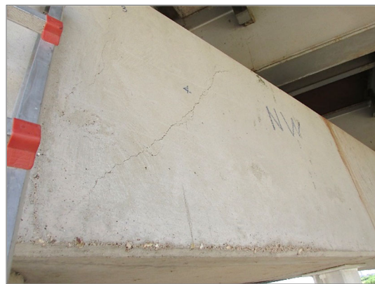
(b) dominant shear crack (northwest face of BC1)
