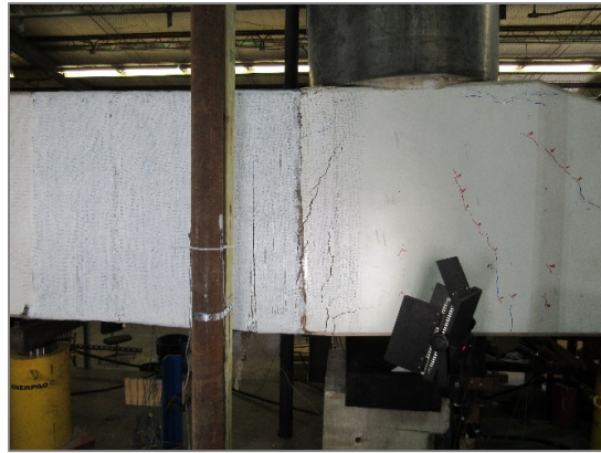
b) Major flexural cracks at the face of the column after reloading (west face)
