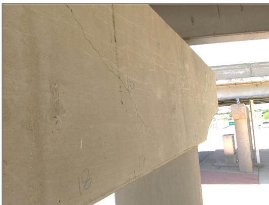
(a) dominant shear crack (southwest face of BC1)
