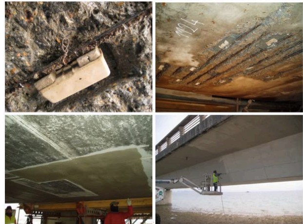
Fig. 6. Details of the repairing procedure (sacrifice anodes, application of mortar patches and final painting)
