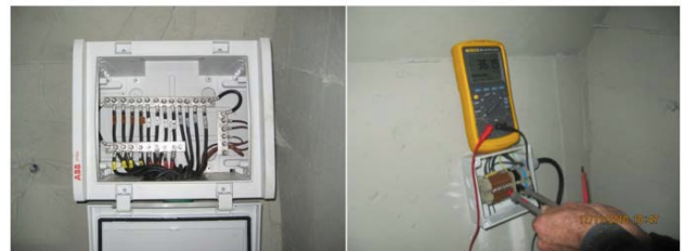
Fig. 9. Detail of a connection box and the procedure of measurement of the voltage
