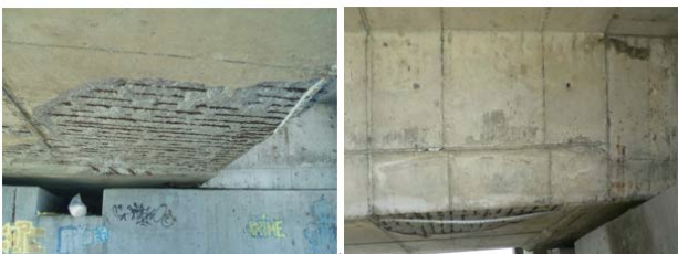
Fig. 5. Affected areas of the bottom of the concrete girder.
