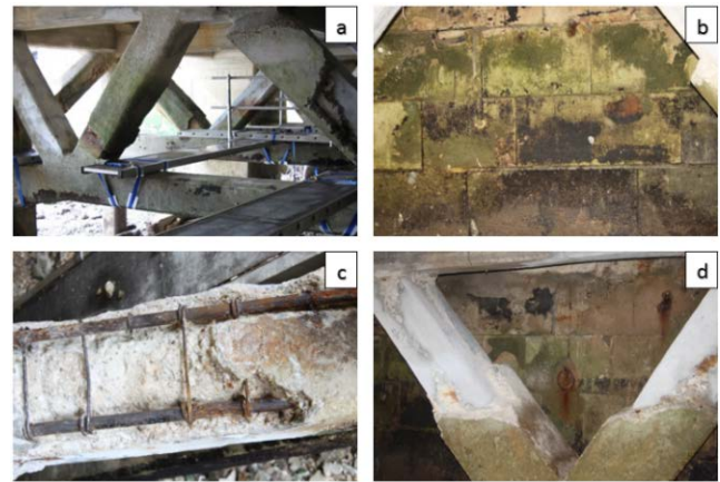
Fig. 2. Deteriorated concrete in the undercroft (Coats et al. , 2015)
