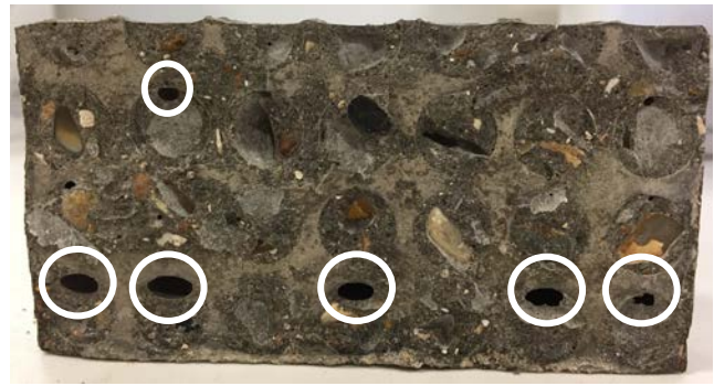
Fig. 10. Air voids at the spacer-concrete interface
