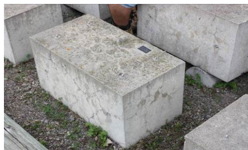
Fig. 2. Disposal of the concrete blocks, i.e. sitting directly on the ground or above ground
