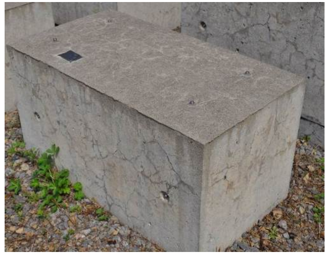
Fig. 12. Condition of exposure block NMLiN1.0 after 15 years outdoors (0.355% expansion)
