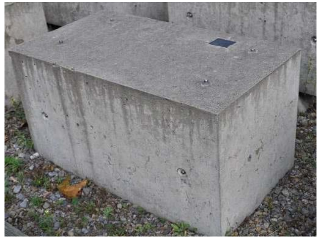
Fig. 13. Condition of exposure block NMLiN1.25 after 15 years outdoors (0.041% expansion)
