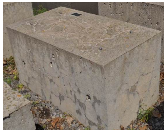
Fig. 18. Condition of control exposure block Wy+ after 15 years of storage outdoors (0.295% expansion)
