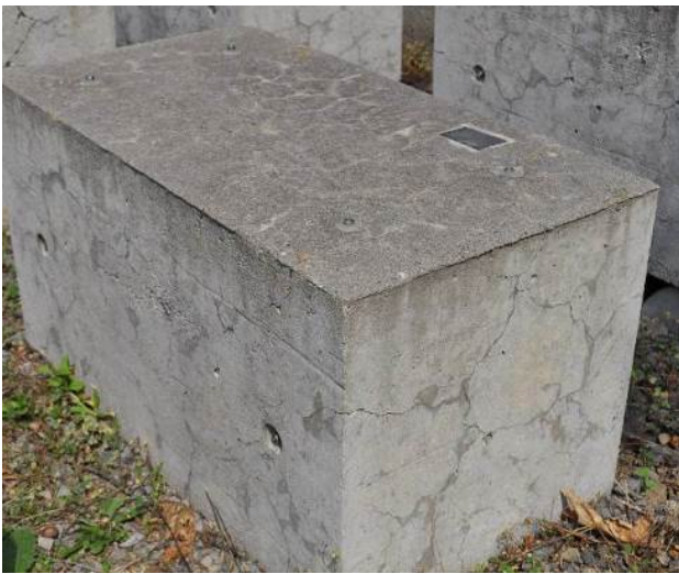
Fig. 10. Condition of exposure block NMLiOH1.0 after 15 years outdoors (0.390% expansion)
