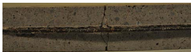
Fig. 11. Example of the opened beam specimen after load-bearing capacity test by three-point bending: cold-worked ribbed steel bar (B7-19), failure by bending. Longitudinal cracking observed. Localised corrosion spots for instance at the crack (crack width w = 0.22 mm)
