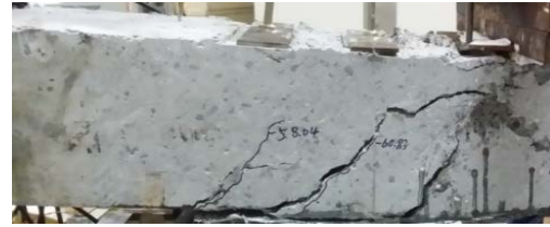
Fig.5. Combined failure of L1500-150-2.
