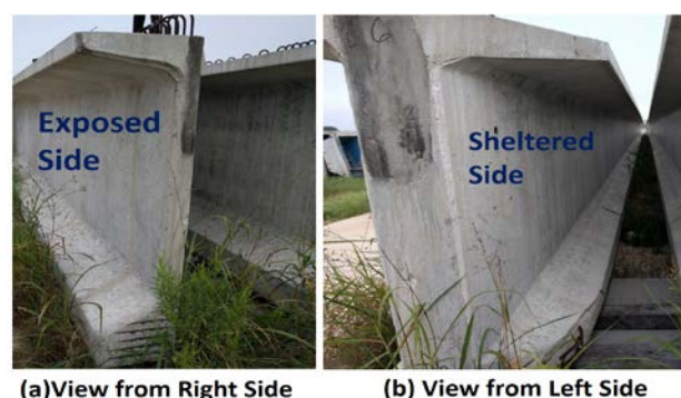
Fig. 2. Photos of a typical rejected girder showing (a) exposed side and (b) sheltered sides
