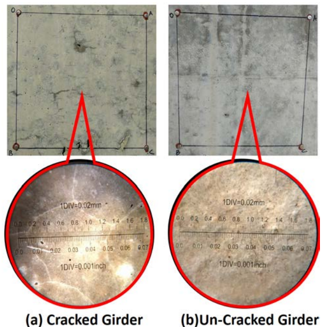
Fig. 6. Typical regions on an (a) extensively cracked and (b) un-cracked girder as visible to the naked eye (top row of photos) and at 50X magnification (shown in the circled call-out)
