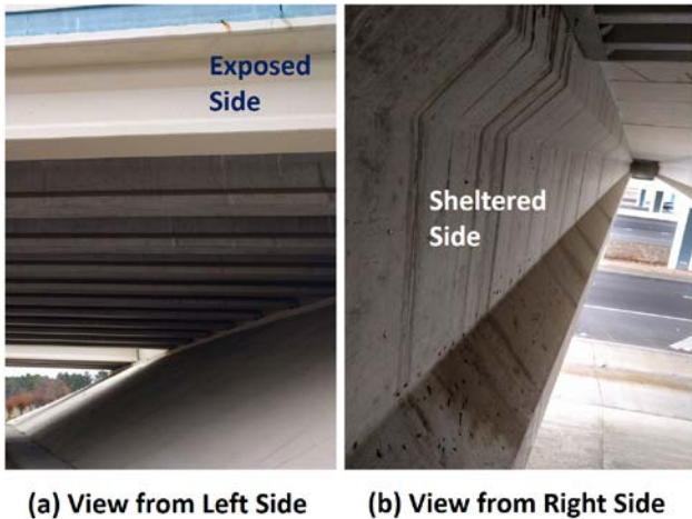
Fig. 5. In-service girder showing (a) exposed side and (b) sheltered side. Notice the exposed girder has been painted.
