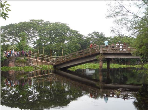
Fig. 1. Silna river road bridge collapse caused by erosion of river bed
