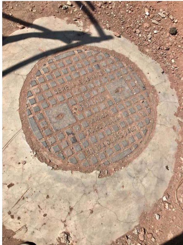
Figure 6. A socio-political take on sanitation governance: the interface of the manhole.
