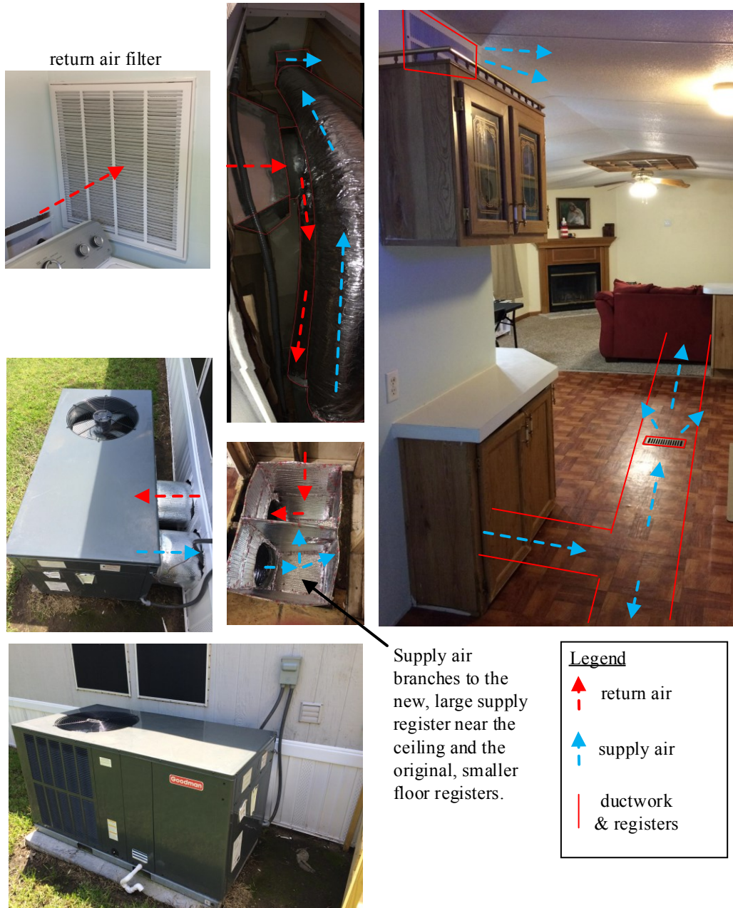
Figure A.2: Several photographs outlining the installation of the HVAC system with the packaged unit, ductwork, return filter, and supply registers.
