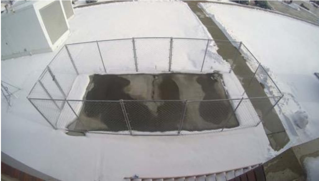
Figure 2.19 Heated test pad after a snowstorm on 27-28 December 2015 [57]
