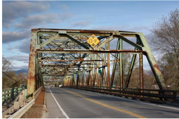
Figure 1.2 Steel bridge highly damaged due to the use of salts to remove ice from the road ( blogs.ei.columbia.edu )
