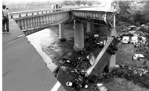
Figure 2. Mianus River Bridge Collapse (from [3])
