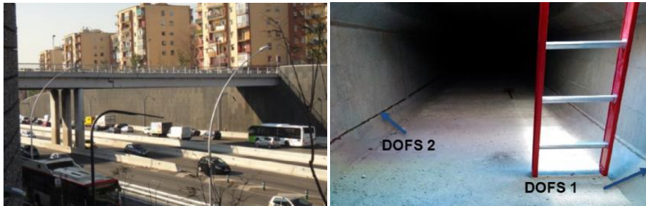
Figure 25. Deployed OBR system in Sarajevo Bridge (Barcelona) (from [46])
