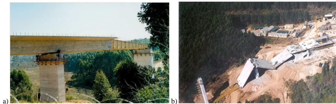
Figure 3. Injaka bridge collapse a) before and b) after (Mpumalangda, 1998) (from [4])
