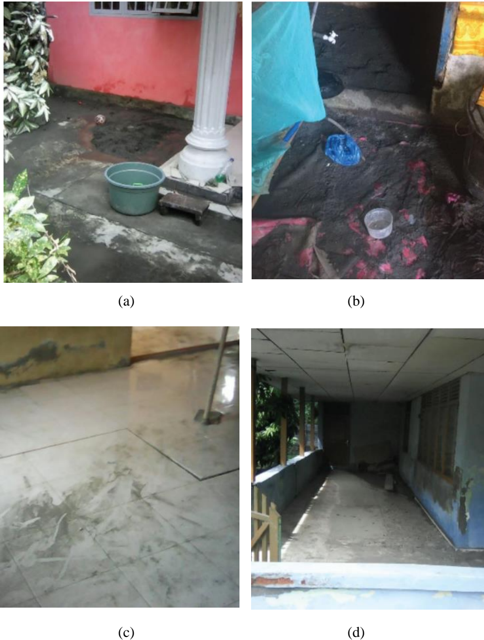
Figure 2. Liquefaction evidence in Pidie Jaya and the surrounding area, (a) boiling sand in local resident, (b) sand boil appears after the earthquake (c) sand boil shown up between tile crack (d) another sand boil evidence in resident area [14]
